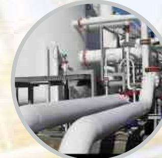
Natural Gas processing
